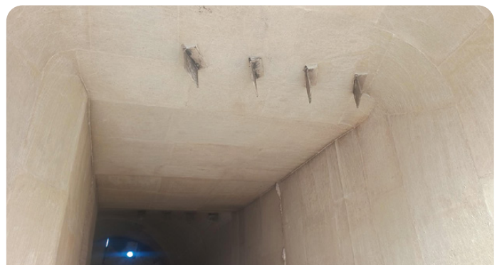
Flue Gas Duct 2
