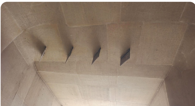
Flue Gas Duct 1
