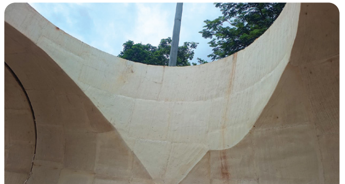
Flue Gas Ducts 2
