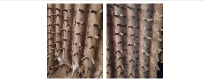
Figure I: Dent, puncture and damages in the water wall tubes when using the traditional way of dismantling
