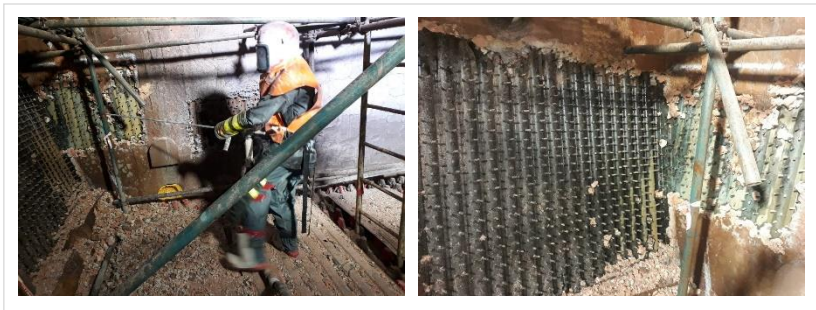
Figure II: Dismantling of refractories by using hydro jetting demolition tools and finished surface
